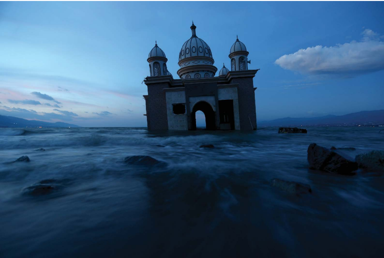
A mosque damaged by the September earthquake and tsunami is seen in a bay in Palu, Central Sulawesi, Indonesia, October 5, 2018. REUTERS/Athit Perawongmetha
